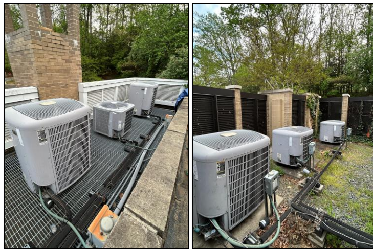
Outdoor Carrier/Daikin Heat Pump Units
