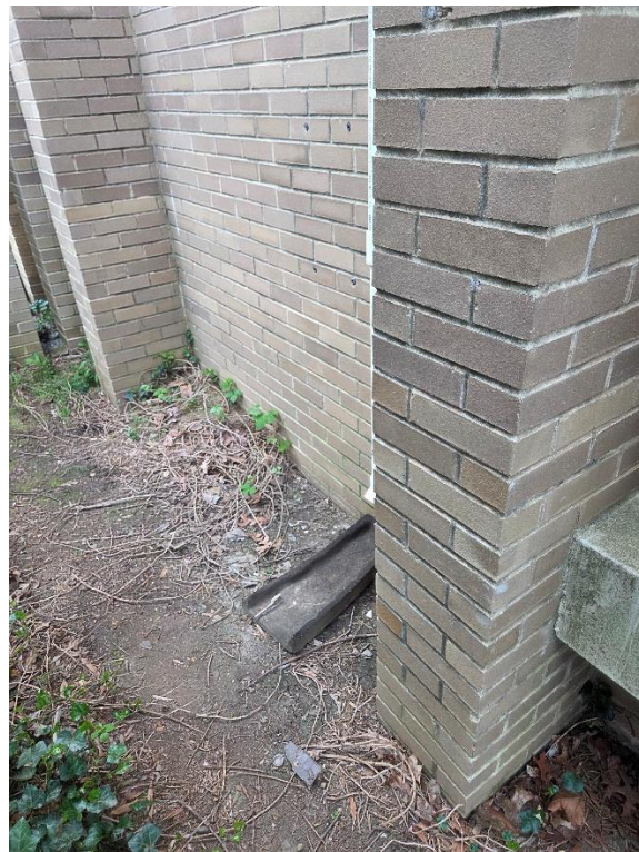
Photo 8: Grade Sloping towards Structure
