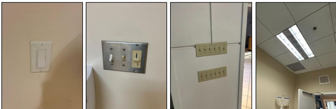
Light Switches and Dimming
