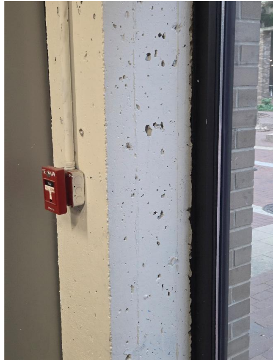
Photo 2: Concrete Column with Surface Pitting
