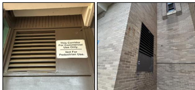
Outdoor Intake Louvers for AHU-5 to 10 (left) and AHU-1 to 4 (right)
