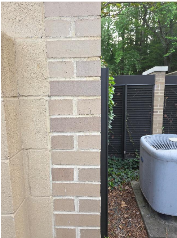
Photo 7: Cracking in Brick
