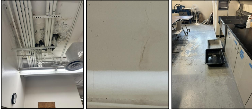
Ceramic Studio Roof Leak
