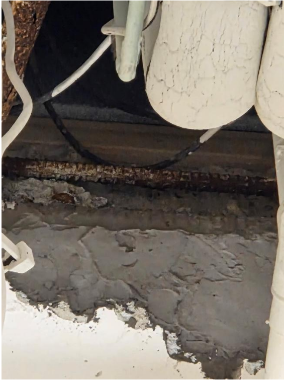
Photo 5: Exposed Rebar in Slab at Penetration
