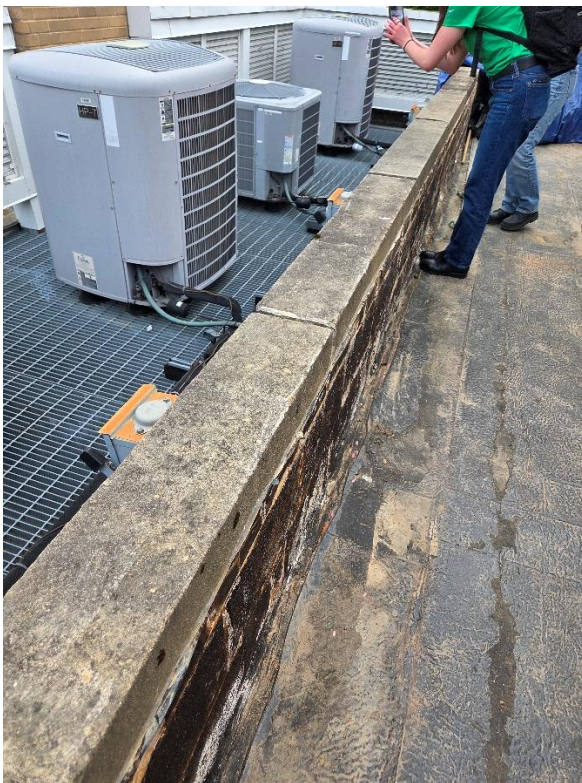
Photo 7: Rooftop HVAC Platform
