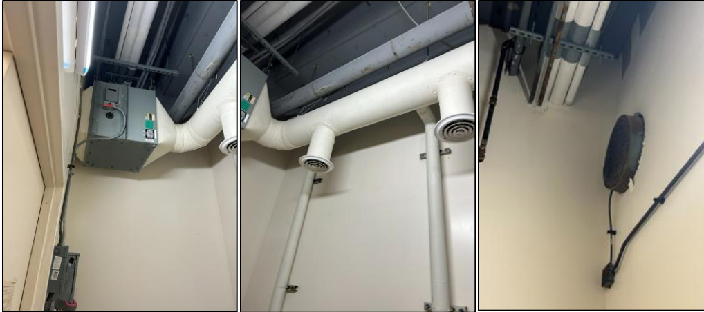
Ducted Powered Exhaust (left and middle) and Ducted Outside Air Connection (right)
