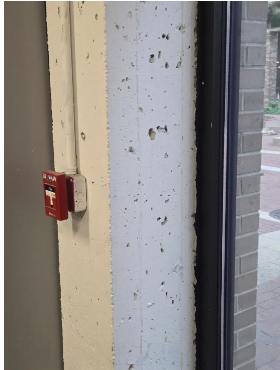
Photo 2: Concrete Column with Surface Pitting
