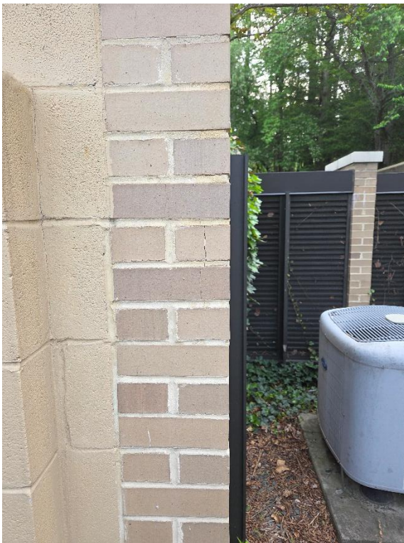
Photo 7: Cracking in Brick
