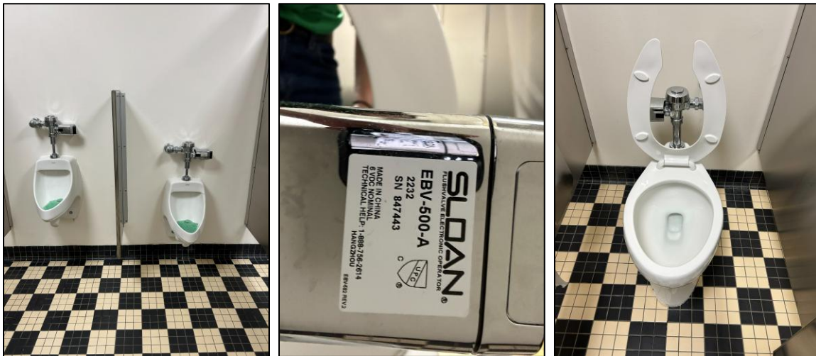
Existing Plumbing Fixtures
