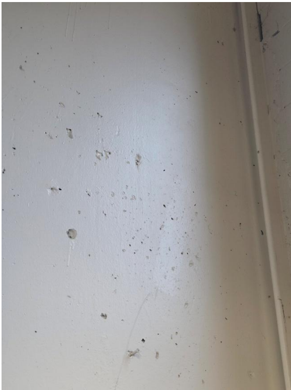
Photo 3: Concrete Wall with Surface Pitting
