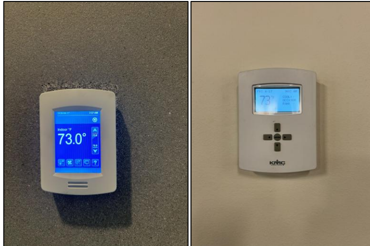
New Thermostat (left) and Older KMC Controls Thermostat (right)
