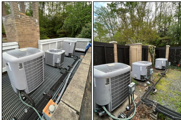
Outdoor Carrier/Daikin Heat Pump Units
