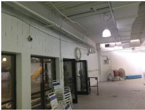
Fig. 40 - Typical CCTV camera
