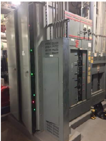
Fig. 35 - Existing MCC, MDP and panel M
