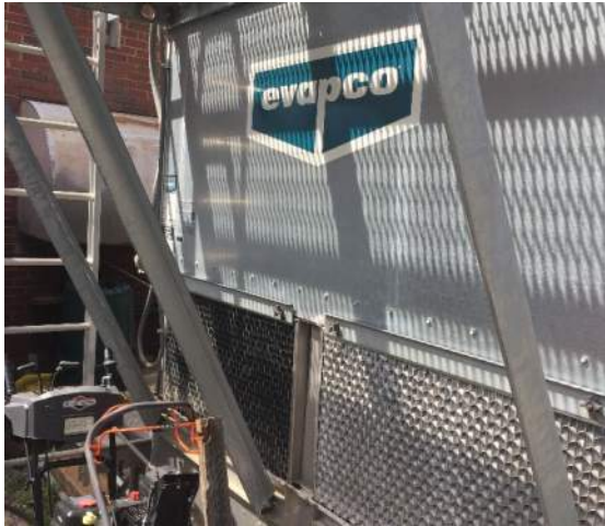
Fig. 34 - Existing cooling tower
