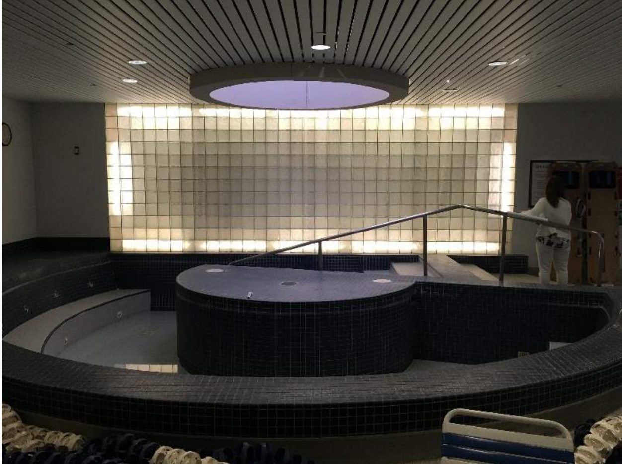
Fig. 25 - Uneven lighting at glass block wall in spa.
