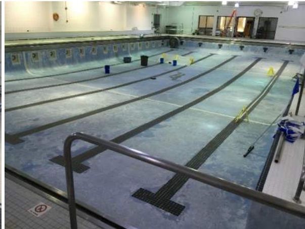
Fig. 23 - Lap lanes drained for cleaning & maintenance
