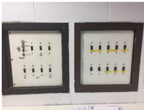
Fig. 43 - Existing lighting control panel
