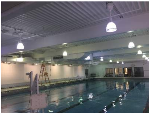
Fig. 41 - Typical pool fixture
